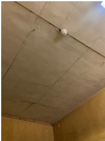
Fig.86: B-22, Cracks to ceiling, most likely a 20th C plasterboard finish.
