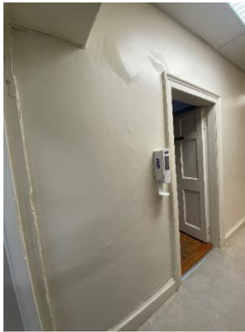
Fig.94: 0-05, paint finish paint finish is lifting from the wall.
