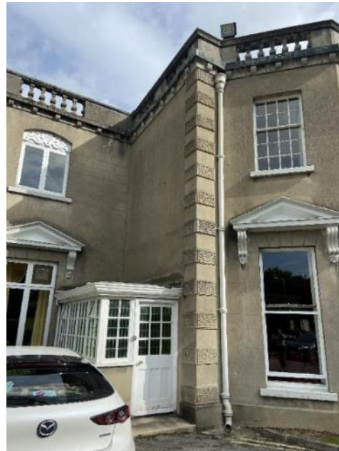
Fig.24: Quoins with vermiculate rustication at junction between early 20th C altered wing and historic core.
