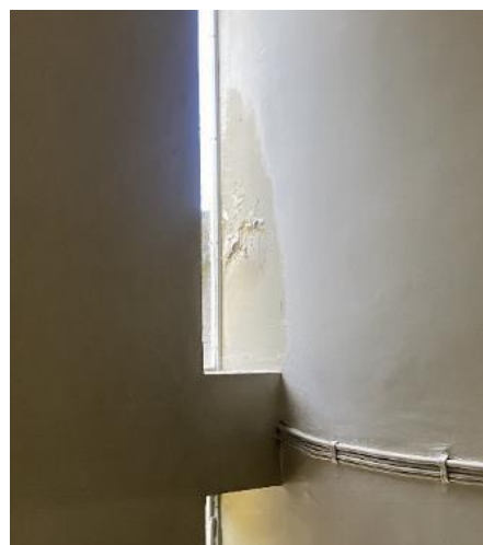
Fig.92: B-09, paint finish is lifting from the wall.
