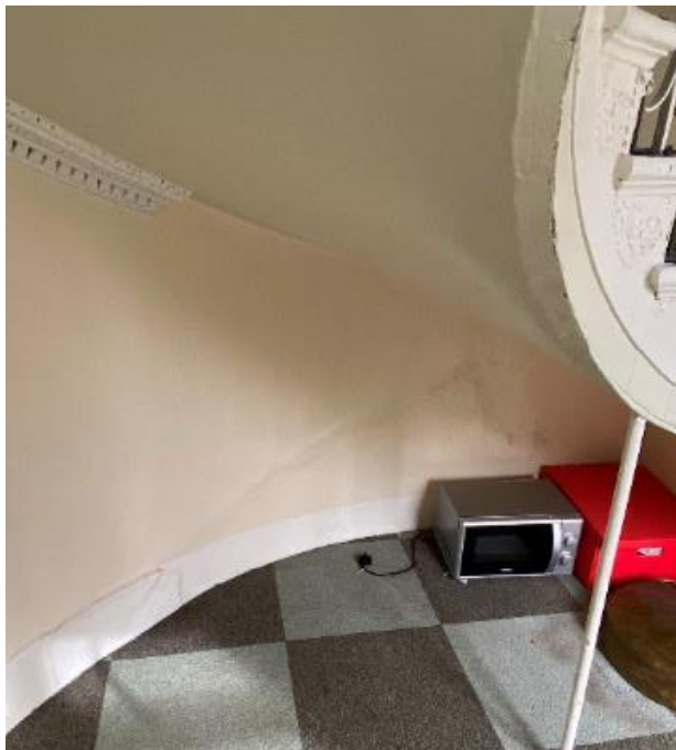
Fig.93: 0-02, plaster is crumbling and coat of paint was applied over it.
