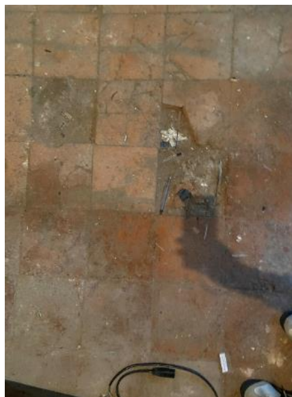
Fig.105: B-23, historic ceramic tiles, missing sections and cracks.
