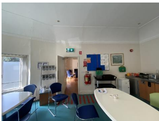
Fig.101: 1-06, Cracks to the west wall
