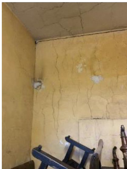
Fig.97: B-22, several cracks
