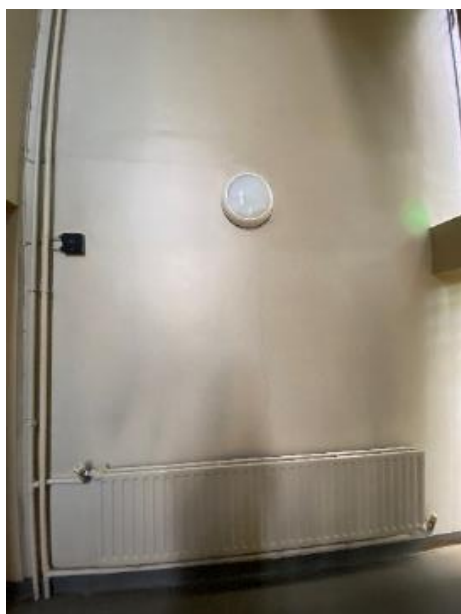
Fig.99: 0-11, Crack to the south wall
