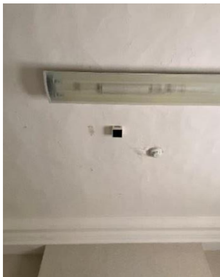
Fig.88: 1-01, Cracks to ceiling.
