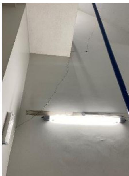
Fig.100: 0-16, Crack to the east wall, south corner
