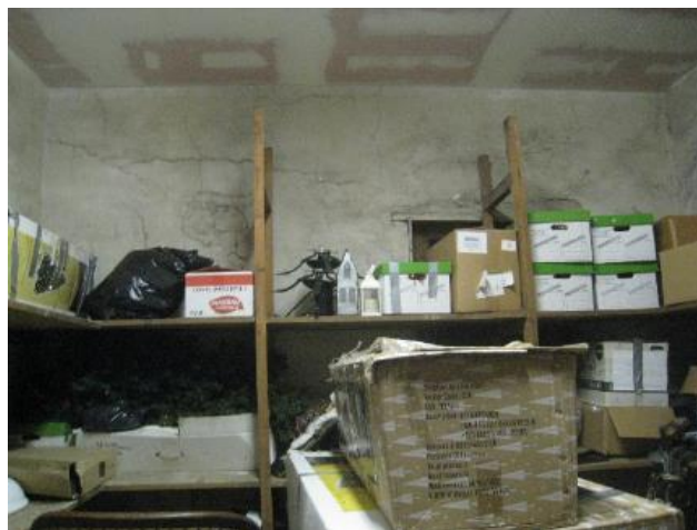
Fig.98: B-38, cracks to the east wall
