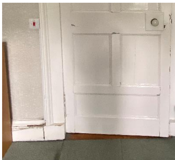
Fig.109: 1-01, historic timber skirting in poor condition
