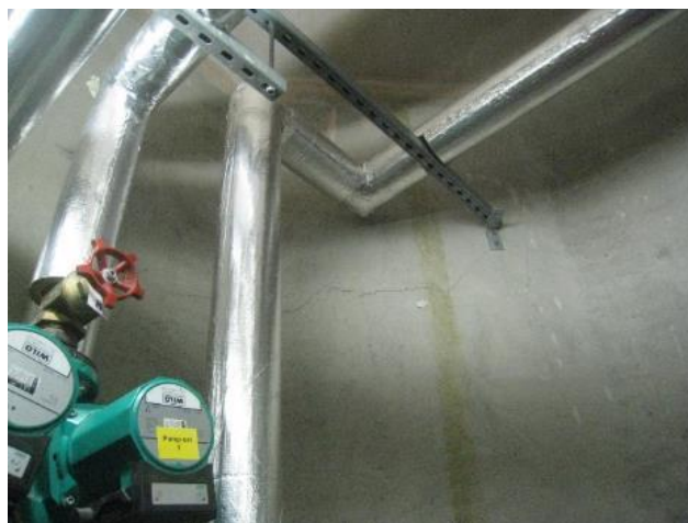
Fig.96: B-37, Inappropriate cementitious render, cracks visible.
