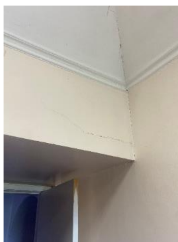
Fig.102: 1-12, Crack running from above door to ceiling
