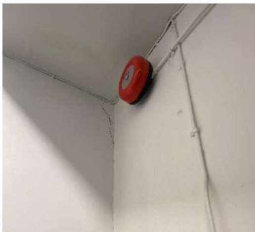
Fig.103: 1-16, Crack to southeast corner wall
