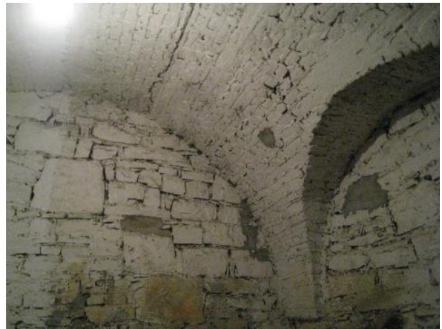
Fig.87: B-39, Crack to brick vault. No works are planned in this room.
