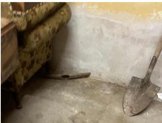
Fig.95: B-22, Inappropriate cementitious render, at bottom section of wall
